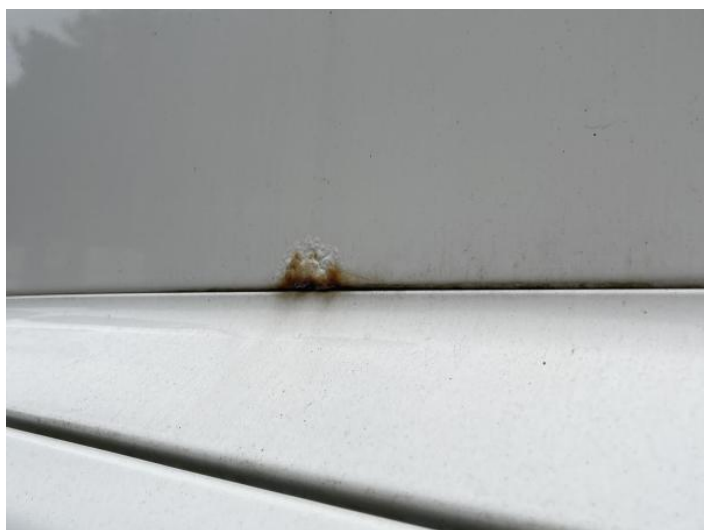
8: Door osf Rusted Over 5mm
